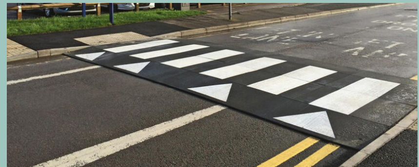
Photo 17. Modular raised crosswalk.
